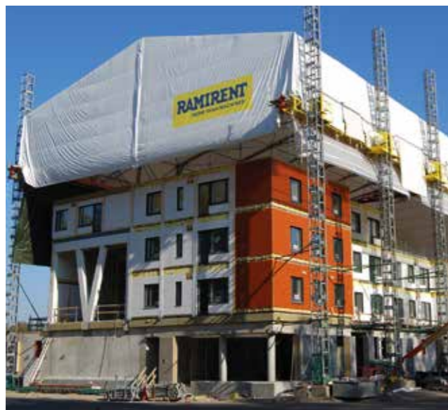
Photo 6. A wooden multi-storey residential building being built for the 2015 Housing Fair in Ylästö, in Vantaa. (Photo: Rakennusliike Reponen)
