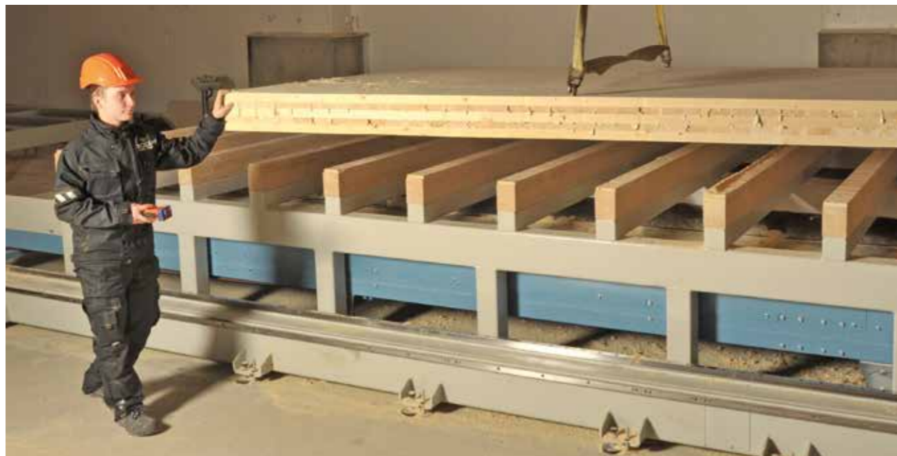
Photo 1. The Finnish company CrossLam in Kuhmo began the domestic production of Cross Laminated Timber (CLT) panels in December 2014. (Photo: CrossLam)
