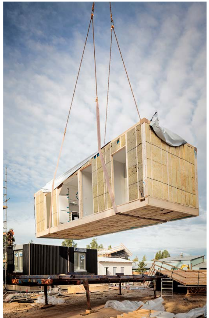
Pre-fabrication in indoor facilities markedly shortens the construction time at the site. (Source: StoraEnso Plc)
