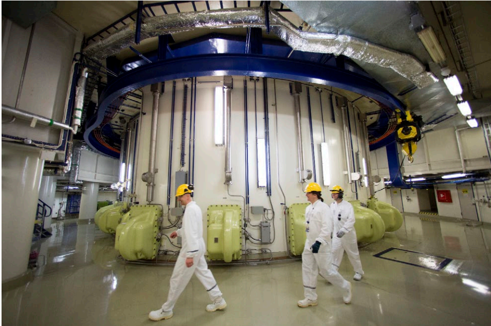
Figure 3.3 Loviisa plant (source: Fortum).
