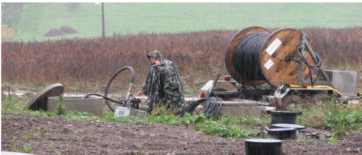
Blowing of an optical fibre cable into a protective pipe installed during the construction of a water supply network (Photo: Network cooperative Kajo)
