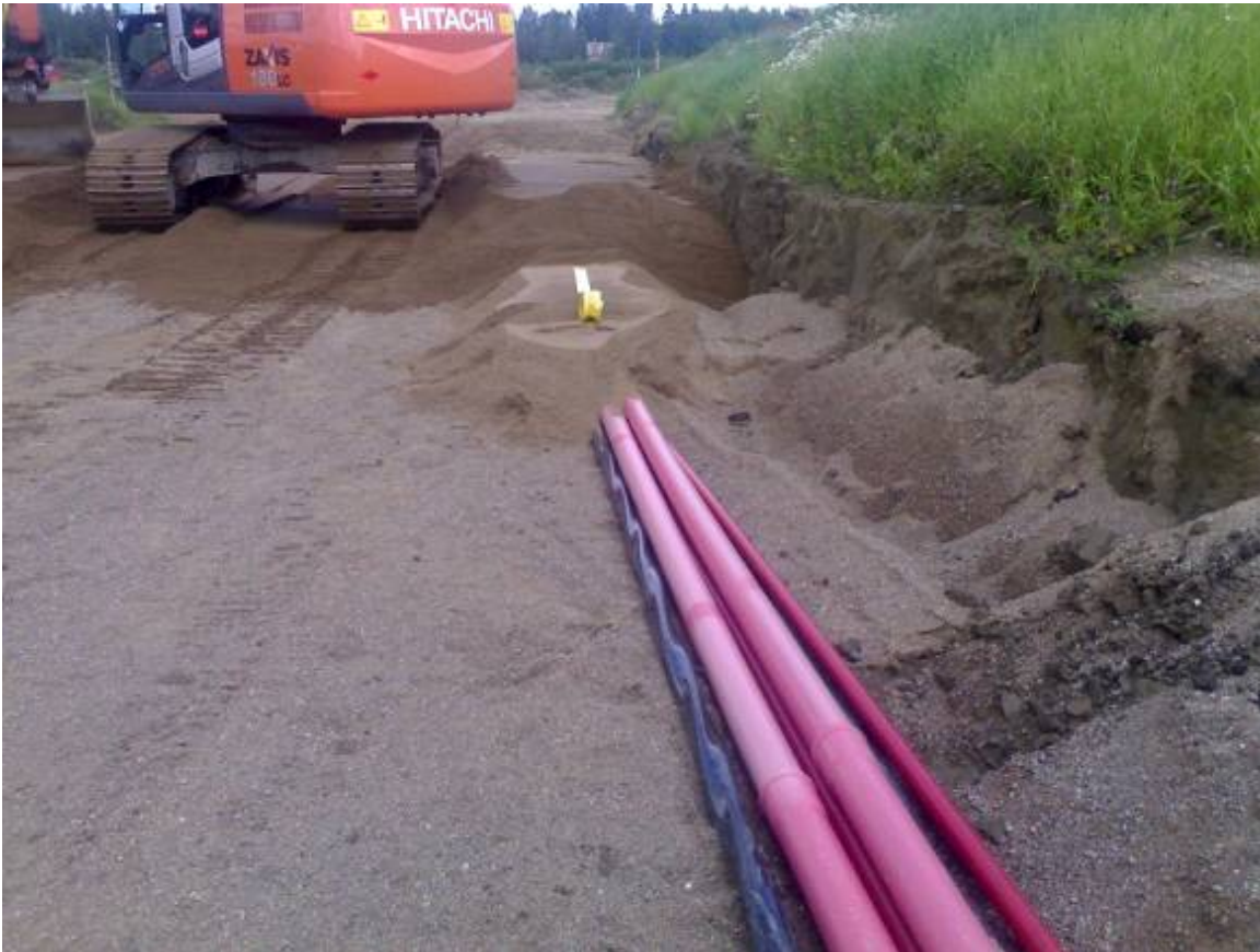
A mid-voltage cable and the piping for a telecommunications cable in a new local detailed plan area in Janakkala (Photo: Vattenfall Verkkö Oy)
