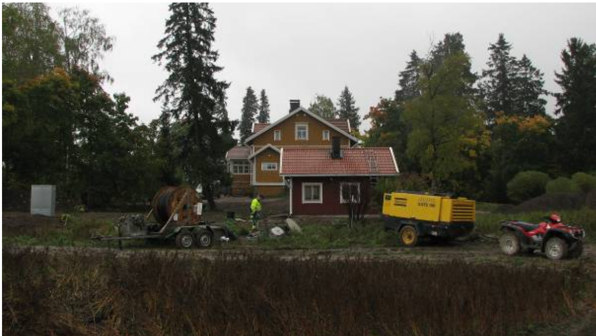
Joint installation of the water supply network and optical fibre cabling. The optical fibre cable is laid inside the installation pipe using the blowing technology. (Photo: Network cooperative Kajo)
