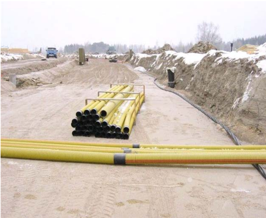
A pipe to be laid under a road and a mid-voltage cable in a new local detailed plan area in Janakkala (Photo: Vattenfall Verkkö Oy)
