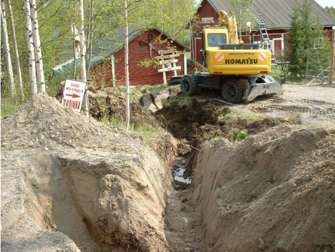
Trench for the optical fibre cable connection of a property (Photo: Reiniko Oy)
